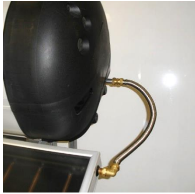
Figure 6-8 Hot Pipe - TS300 Open Circuit
